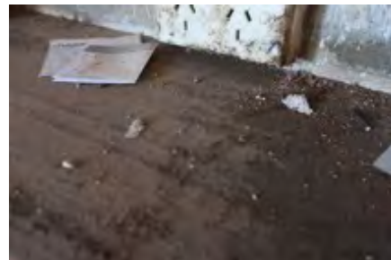
Debris in cabinet
