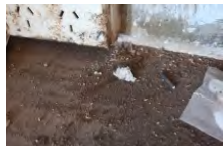
Debris in cabinet
