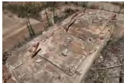
Debris on Ground
