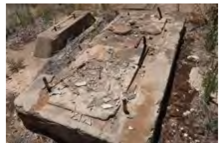
Debris on Ground
