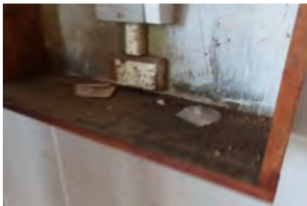
Debris in cabinet
