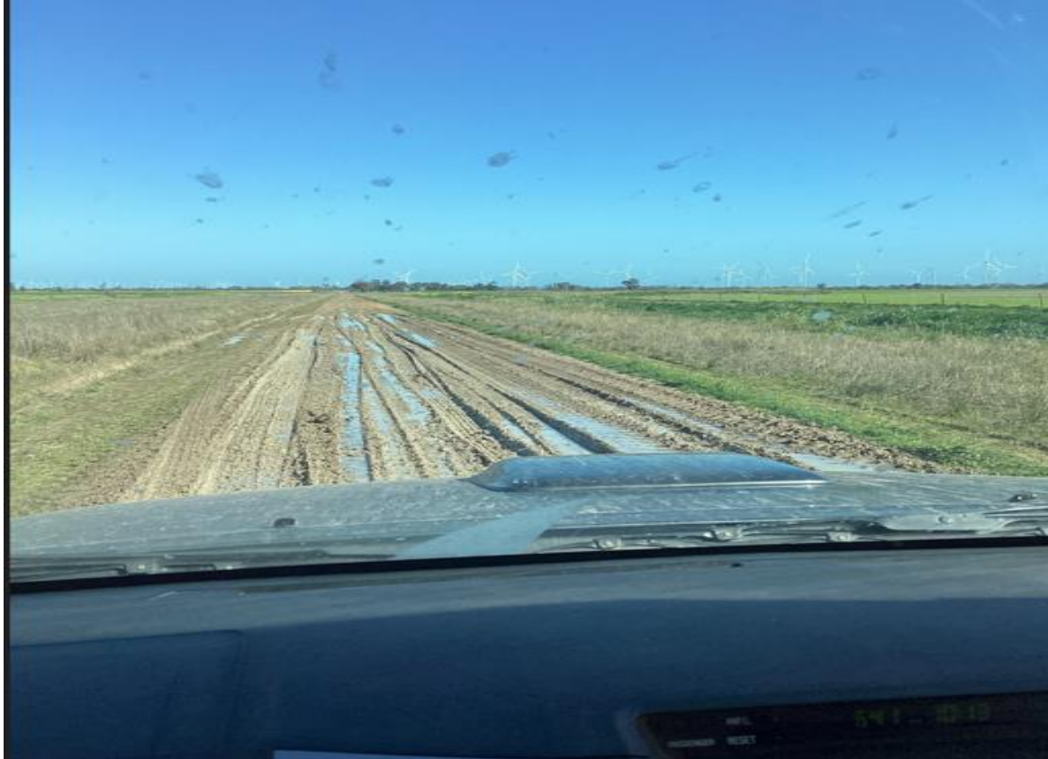
Picture 3 Road condition of Yarriambiack Drive
