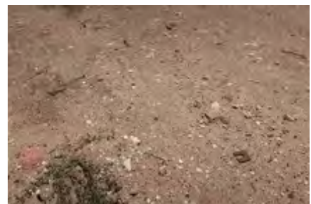
Debris on Surface
