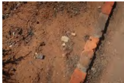
Debris on Surface
