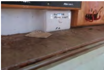
Debris on Surface
