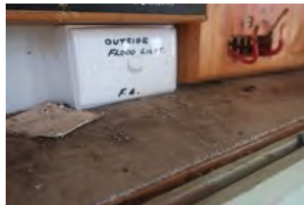
Debris on Surface
