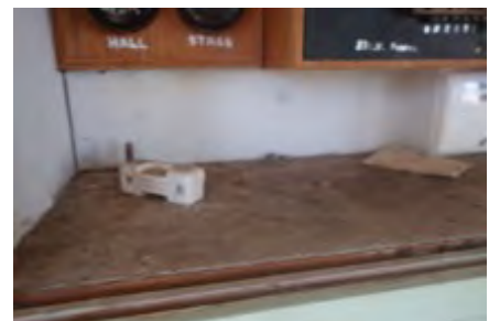
Debris on Surface
