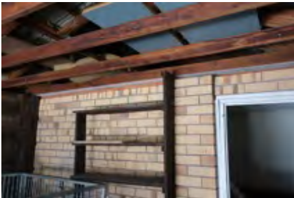
Maintain paint or sealant
