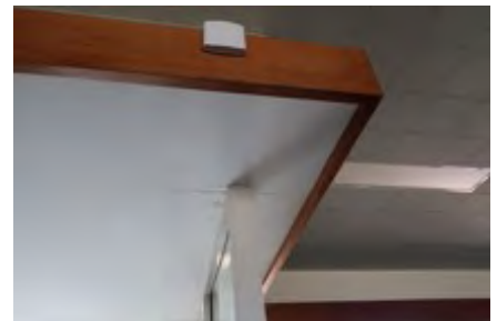
Maintain paint or sealant
