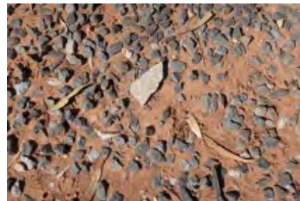
Debris on Surface
