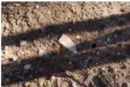
Debris on Surface
