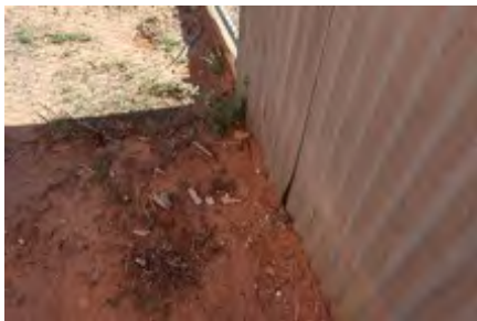
Debris on Surface
