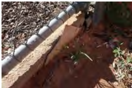
Debris on Surface
