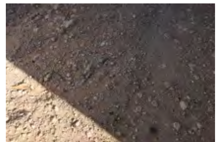
Debris on Surface
