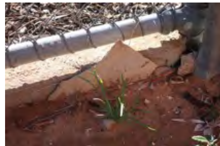
Debris on Surface
