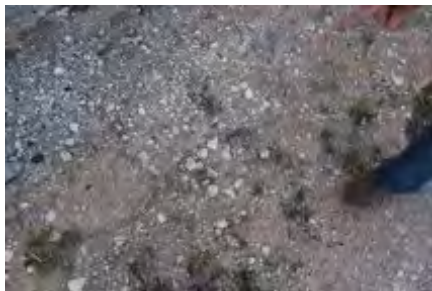
Debris on Surface
