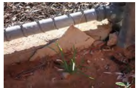
Debris on Surface
