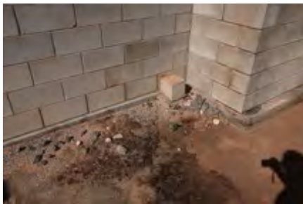
Debris on Surface
