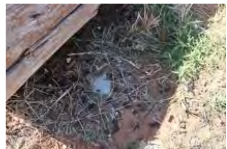
Debris on Surface
