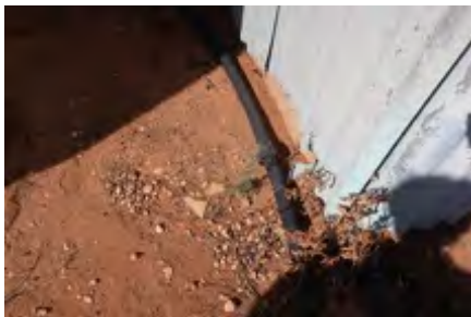
Debris on Surface
