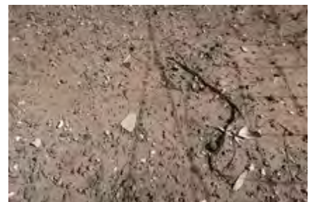
Debris on Surface
