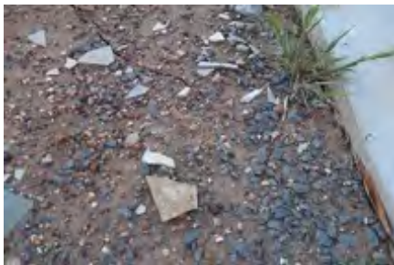
Debris on Surface
