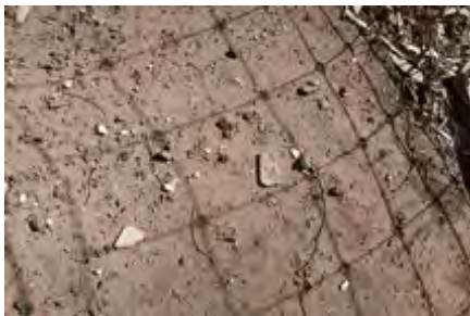
Debris on Surface
