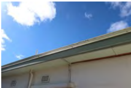
Maintain paint or sealant
