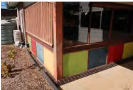
Maintain paint or sealant
