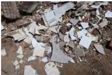
Debris on Surface
