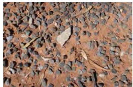
Debris on Surface
