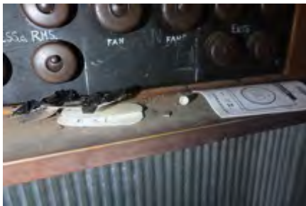
Debris on Surface
