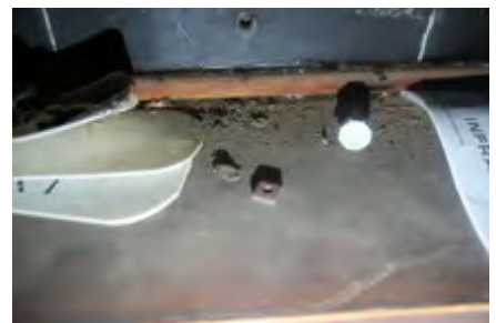
Debris on Surface
