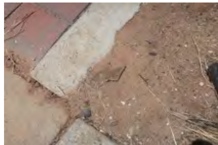
Debris on Surface
