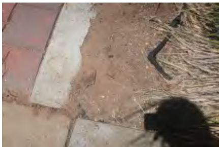
Debris on Surface
