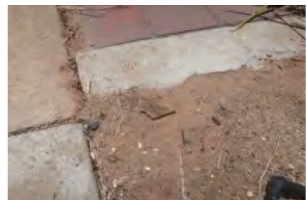
Debris on Surface
