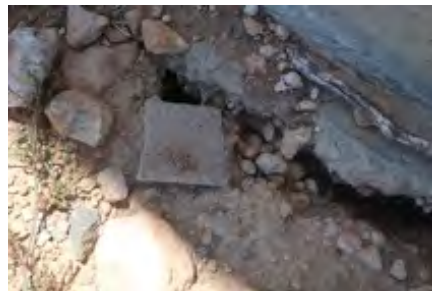
Debris on Surface
