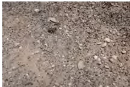
Debris on Surface
