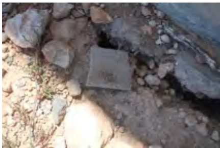
Debris on Surface
