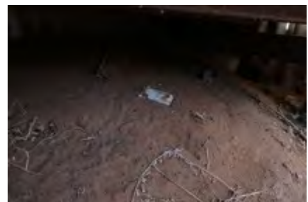
Debris on Ground
