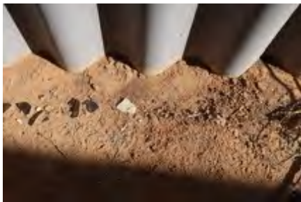
Debris on Ground
