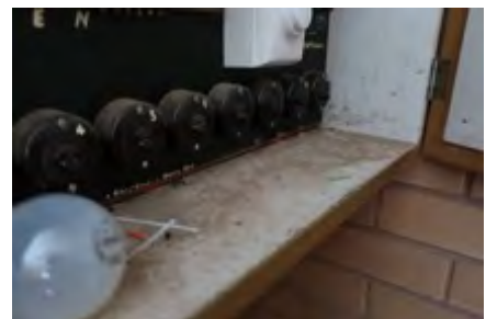
Debris on Surface
