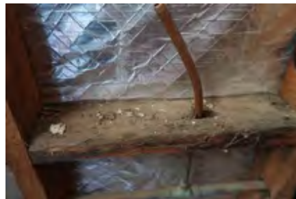
Debris on Framing
