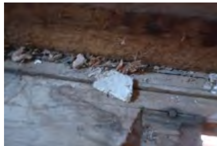
Debris on Floor
