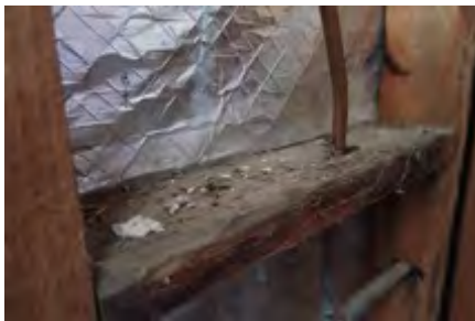
Debris on Framing
