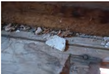
Debris on Floor
