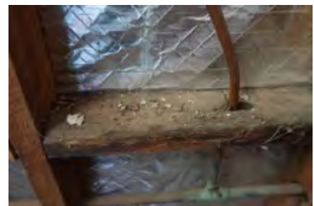
Debris on Framing
