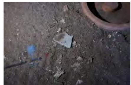
Debris on Ground
