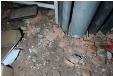
Debris on Ground
