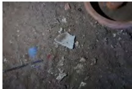
Debris on Ground
