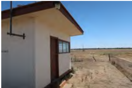
Maintain paint or sealant
